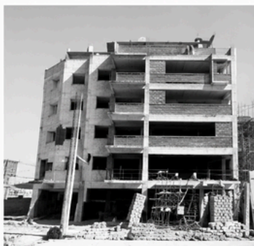
The Pancake Collapse- Soft Storey Failure
