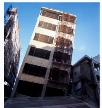
The Soil Liquefaction Lie- Foundation Failure
